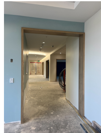
NW 3rd Floor Corridor Doorway Jams
