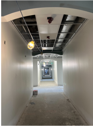
SW 3rd Floor Corridor Lighting/Device
