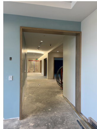
NW 3rd Floor Corridor Doorway Jams
