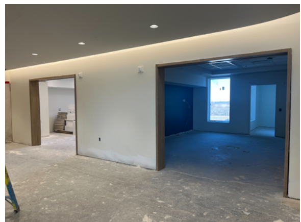
NW 3rd Floor Care Centre/Sun Room Door Jams
